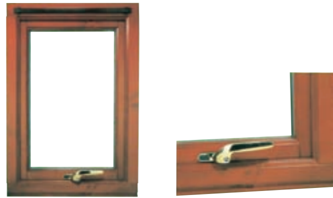
Internal view showing mould on both sash and frame. (Note: non-standard brass handle is shown).
